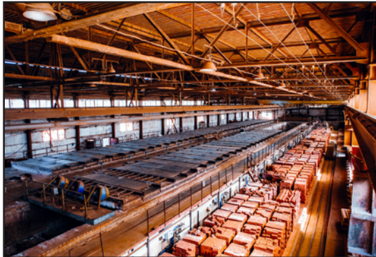
Brick conveyor chains failing due to residue buildup.
